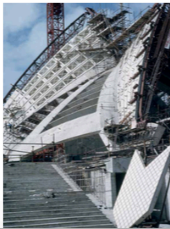
17 Precast concrete panels are assembled on the ribs of the Sydney Opera House (1958–73), c. 1966. Ove Arup's team used early computers to analyse the complex shell structures.
